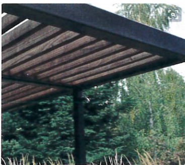
8. OVERHANGS: Natural wood trellis- 4x12 douglas fir beams with clear polyurethane finish
