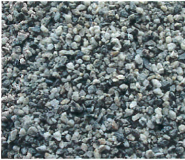
1. ROOFING: Class A type 4 ply built up roofing finished with granite No. 5 1/4" by A1 Grit CO.
