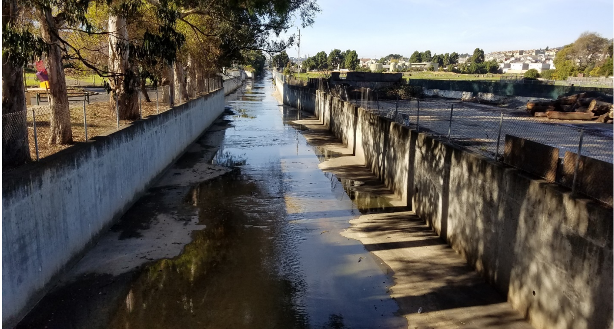
Figure 3-4. A shift in the Colma Creek alignment, looking upstream to the confluence with 12 Mile Creek.
