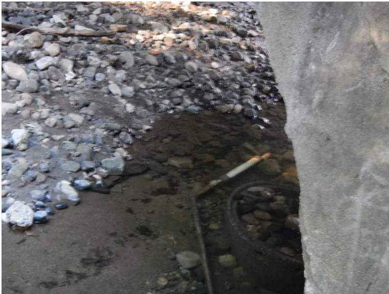
Figure 3: Suction Piping in Alpine Creek
