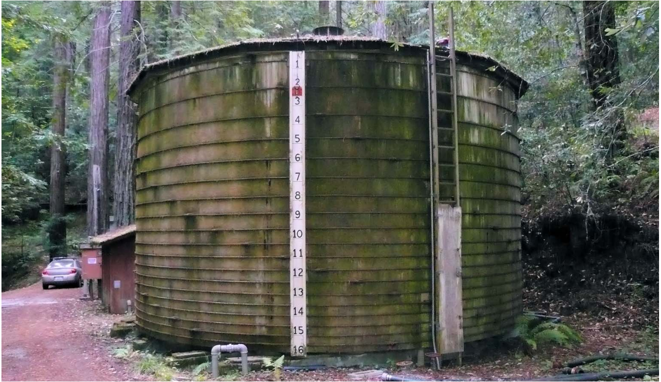
Figure 7: Raw Water Redwood Tank & Inlet/Outlet Pipe Connection
