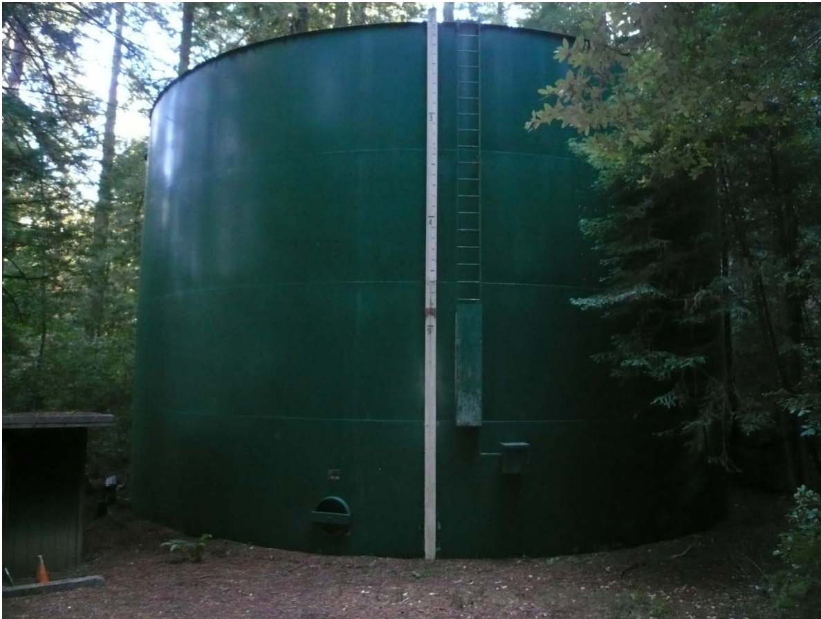
Figure 8: Treated Water Tank & Inlet/Outlet Pipe Connection
