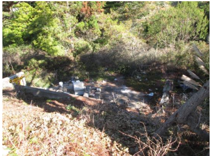
20. View of a concrete building pad with various debris on the subject property
