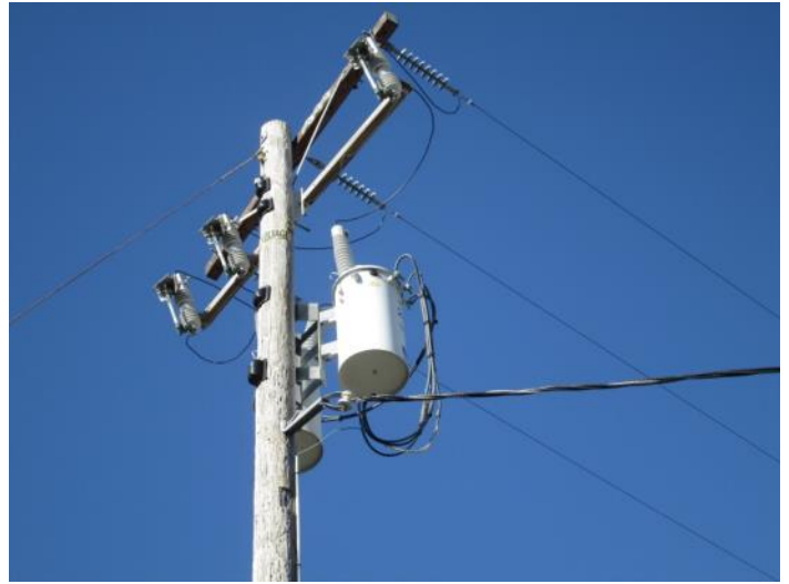
18. View of pole-mounted transformer and power lines on the subject property
